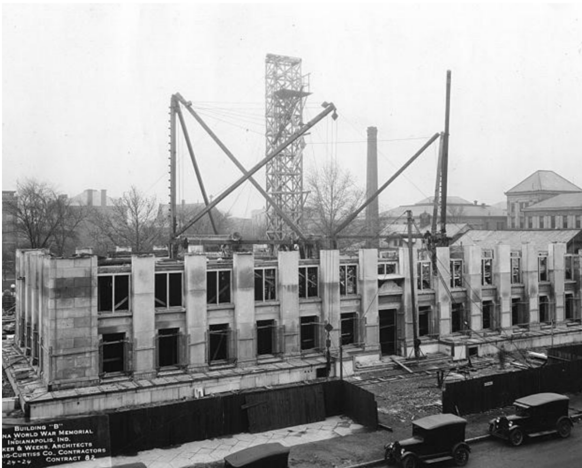
Construction of Building "B". The original national headquarters of the American Legion and associated organizations, November 1924. War Memorials Commission.
